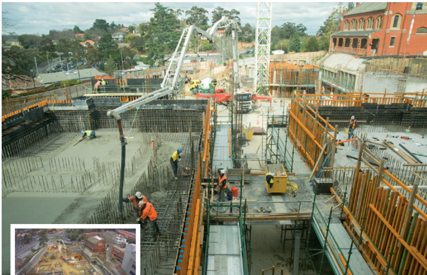
Construction of the radiation bunkers are well on their way. Photos courtesy of Peta Philips.
