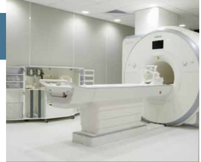
Pictured here is the new 3 tessa MRI machine. This eight tonne machine was lowered into the building after the cleverly designed roof was lifted off.
